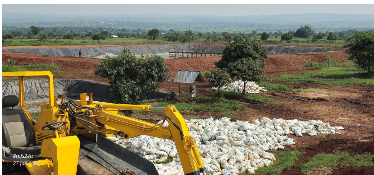
Figure 7: Run of Mine Stockpile & Tailings Storage Facility - Mwamba Processing Plant, Tanzania ©Mwamba
